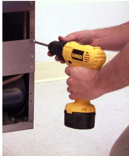
Removing gas manifold shield.
